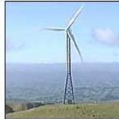
A wind turbine
